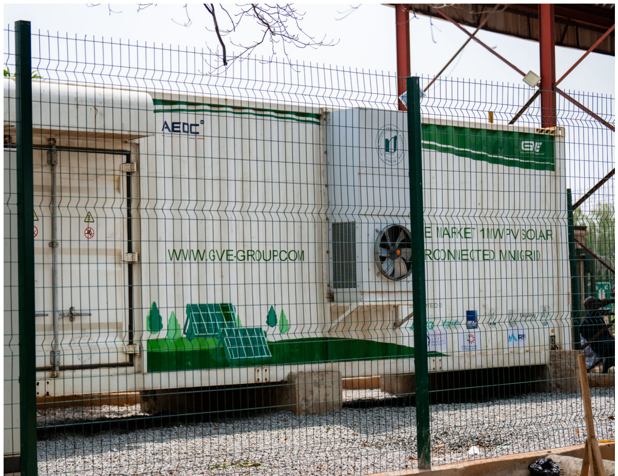
BESS in Wuse IMG.
