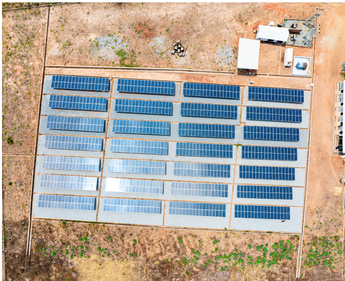
Toto IMG generation plant.
