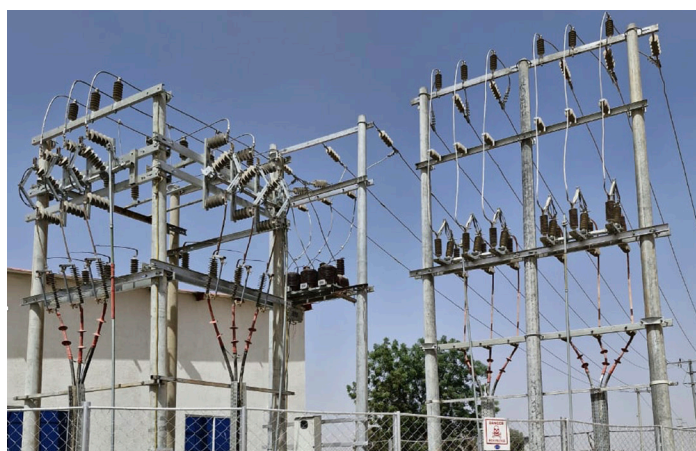
Interconnection point of the Zawaciki IMG, showing the incoming 33 kV line with its associated current transformer and energy meter.
