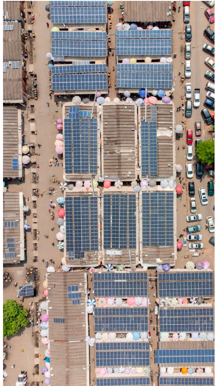
PV modules on top of stalls at Wuse IMG.
