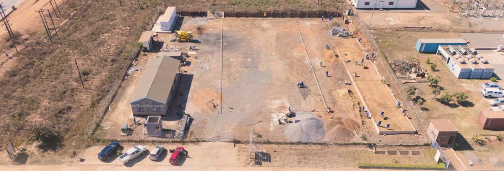
Workers in Malawi prepare the Lilongwe site for the new batteries. The grey building on the left houses soon-to-be-decommissioned diesel generators. Photo: Global Energy Alliance
